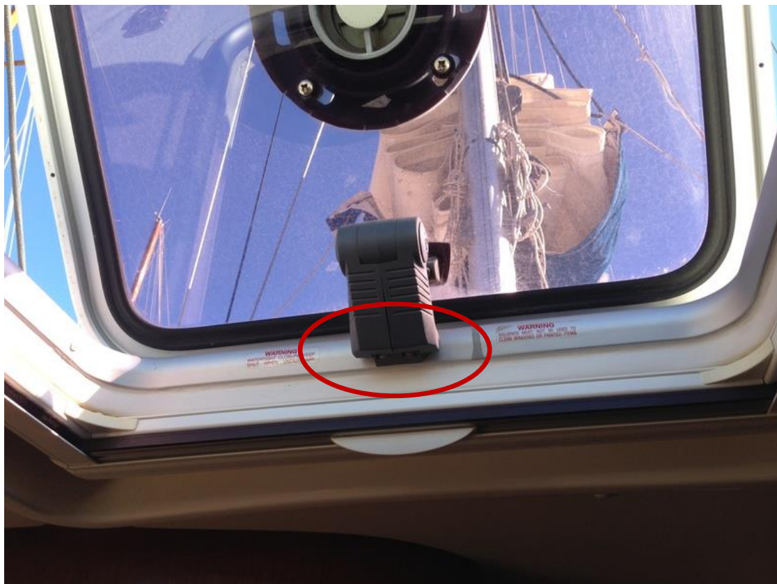
Shown place of hatch supporting rivets were not tight enough. In time they will loosen much more.
