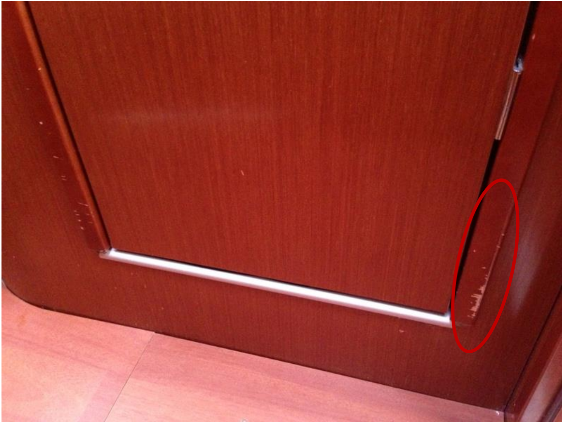
Cosmetic defects on saloon.
