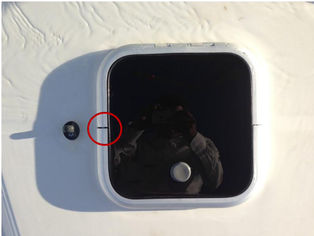
Detachment was seen on starboard side hatch that was located on coach roof.
